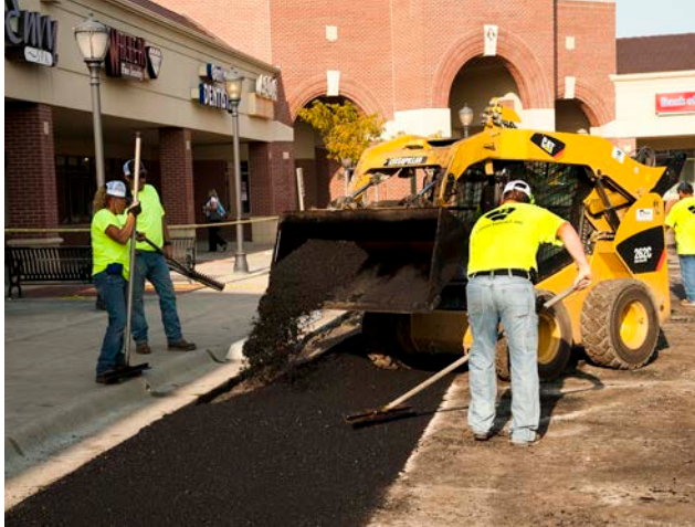
K.A.I. Total Pavement Management delivers customized asphalt maintenance, repair and reconstruction services to all types of businesses across the US.
